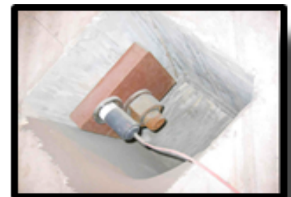
Fixed Position Vibration Sensor
